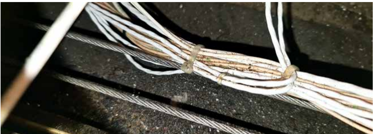
// Wiring bundle attached to a flight control cable – note the metal shavings on the wire.
